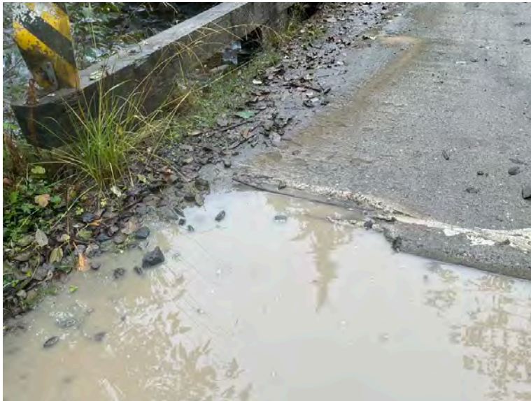
Left bank ballast wall and panel damage
