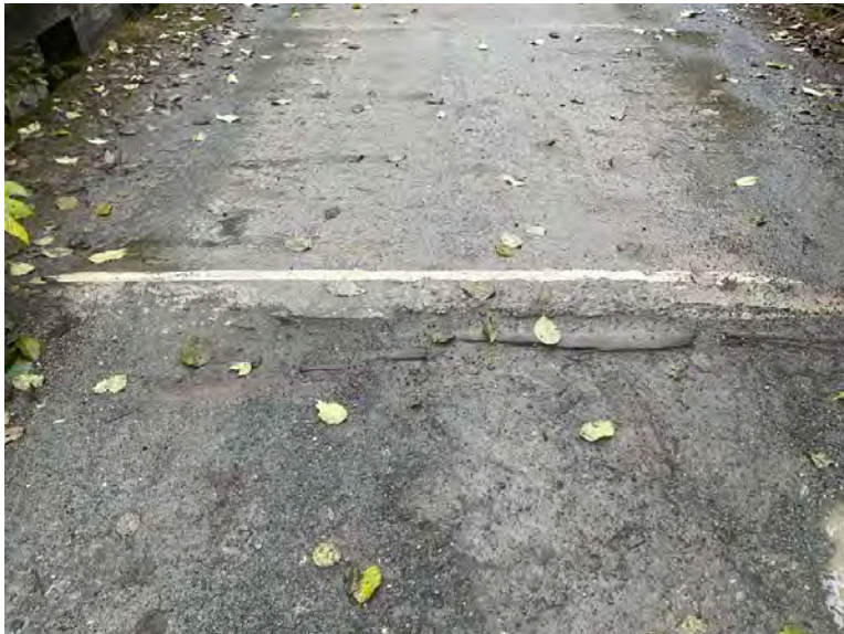
Right bank ballast wall damage
